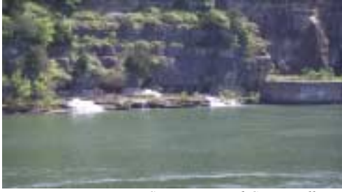
Seepage around Center Hill Dam
